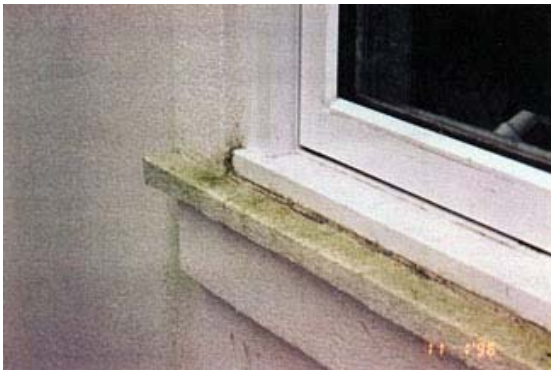
Cracking on window joints (above)
