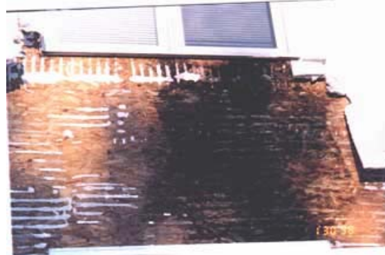
Resulting water damage from failure (above)
